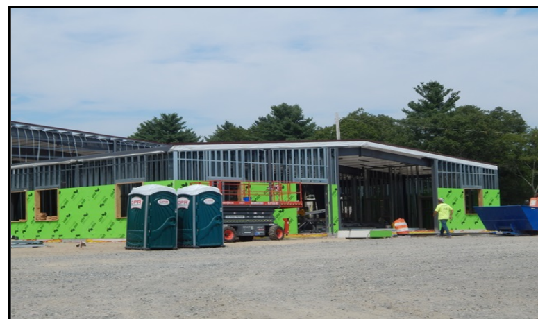
Metal Stud Framing and DensGlass Sheathing Installation in Admin Area. Window Openings Established.
