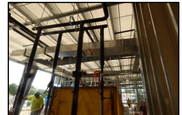
Piping for Boiler Room.
