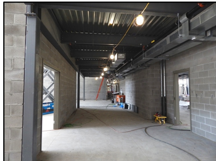
Interior Garage Area CMU Walls Under the Mezzanine. Sprinkler & HVAC System Piping.
