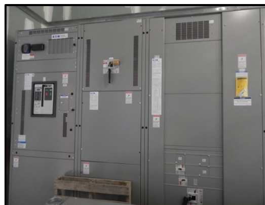
Interior Electrical Service Main.
