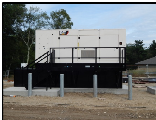
The New DPW Building Generator.
