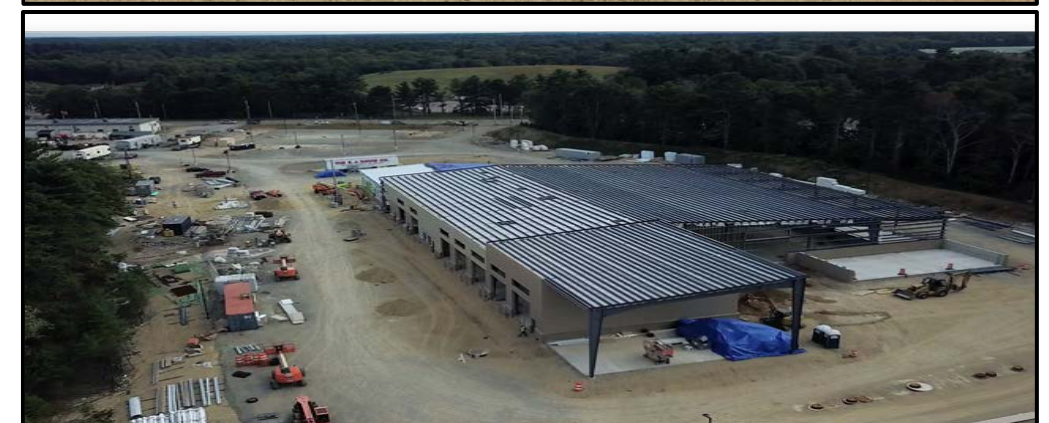
Top: Garage Area Siding Installed / Bottom: Looking South - Drone View of the Site.
